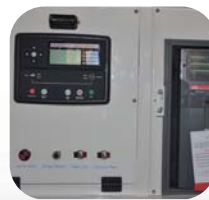
Control Panel & MCB
